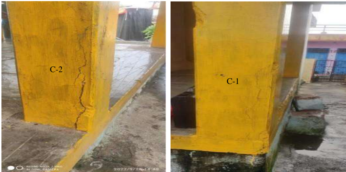
Fig 5: Column with major cracks
